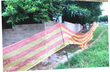
Our rather rickety "security fence" is well on the way to being somewhat more secure.
