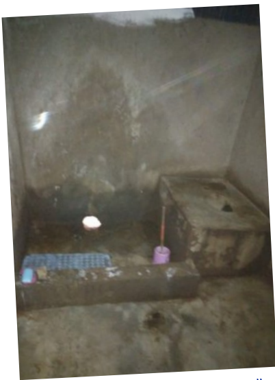
The current "bathroom"
