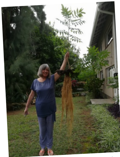
This plant was growing out of our reserve water tank
